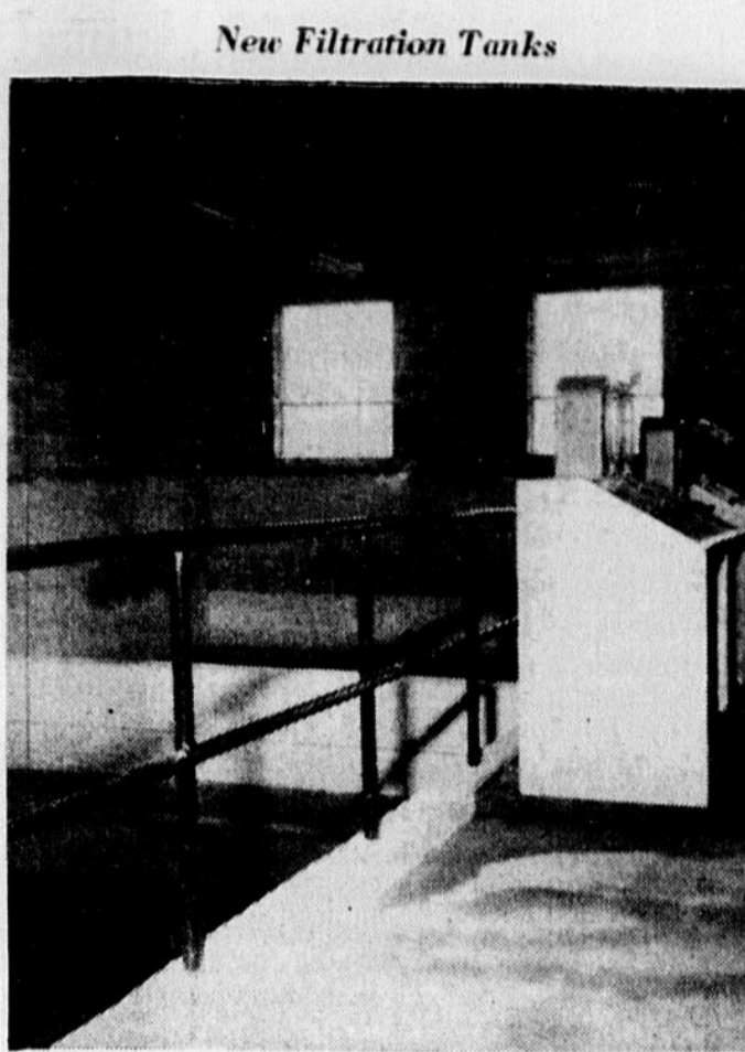
These are the two new filtration tanks which form a major part of the recently installed equipment. Each tank is capable of handling up to 500,000 gallons of water daily. The consoles in front give automatic readings on the rate of flow of the water through the tanks and the amount of dirt in the filters. In addition, the consoles are equipped with hydraulic controls for opening and shutting valves. Filter tanks are cleaned about three times a day by reversing the flow of water through them. See article for explanation of the filtering system.
