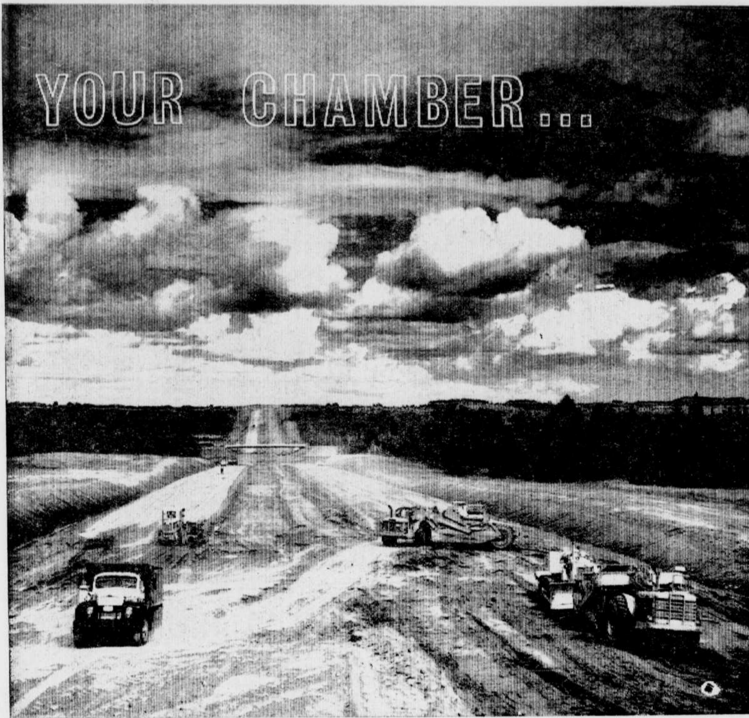
EASTERN TOWNSHIPS AUTOROUTE — This view shows construction of the Eastern Townships Autoroute near Cherry River. (Record photo by Doug Gerrish)
