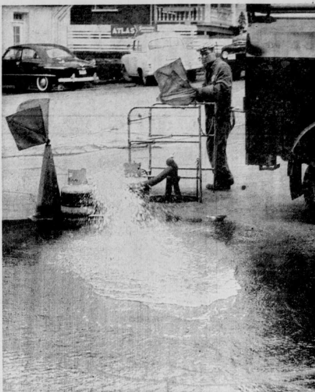
FLOODED MANHOLE — A flooded manhole on the corner of Wellington and Aberdeen Streets in Sherbrooke had to be pumped by the Bell Telephone Company Tuesday afternoon before a repair man could descend to fix a new cable. Above, water spurts from the manhole while a Bell man looks on. (Record Photo by Gerry Lemay)
