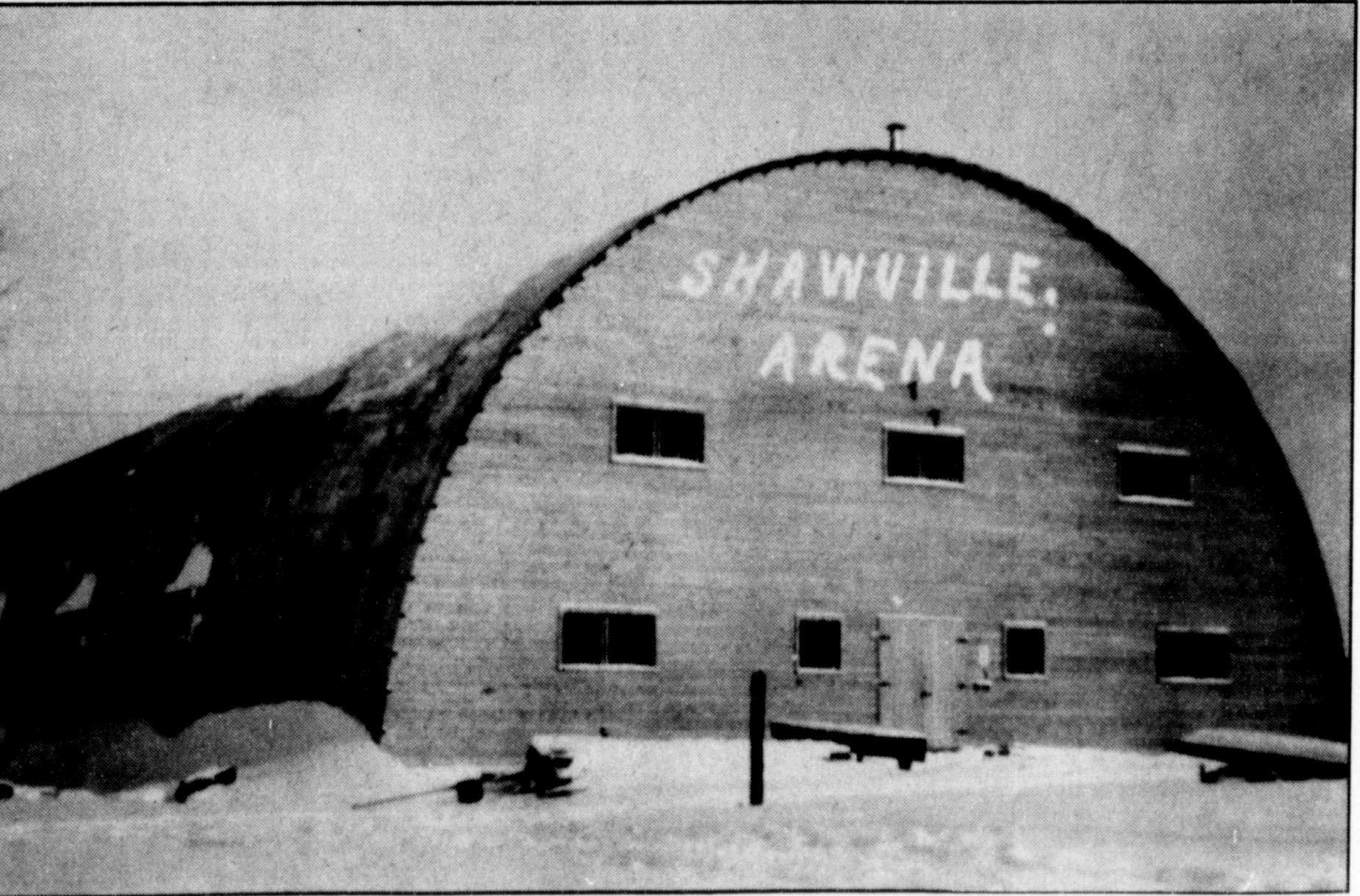
Heavy snow forced the Richardson Rink to cave in during the winter of 1972.
