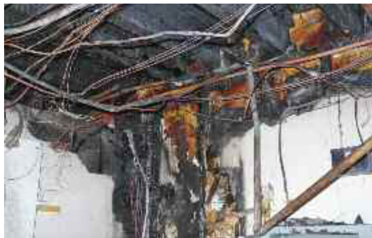
The origin: electrical distribution system.
