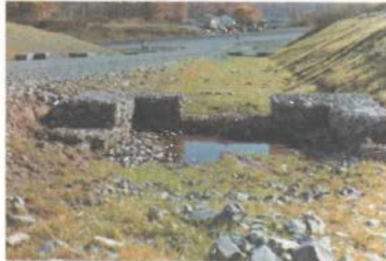
A properly installed series of gabion check dams. Note also the effectiveness of hydroseeding and lining the ditch with rock to achieve maximum erosion control.
