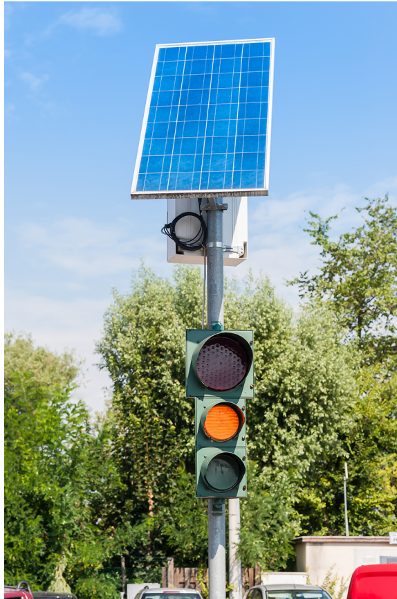
Figure 21. Solar-power traffic lights.
