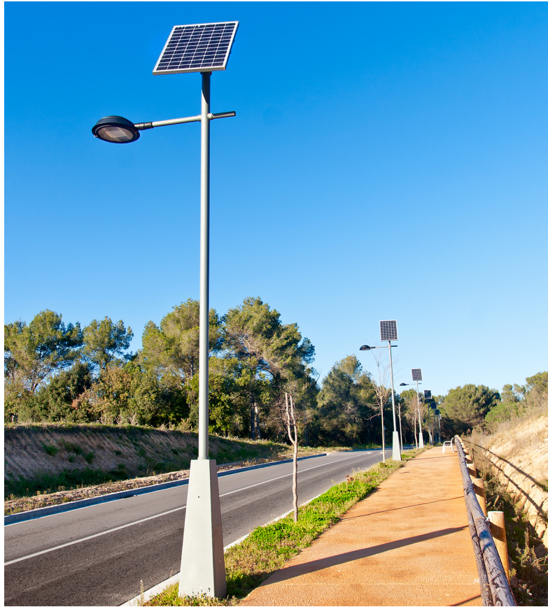
Figure 20. Solar-power street lighting system.
