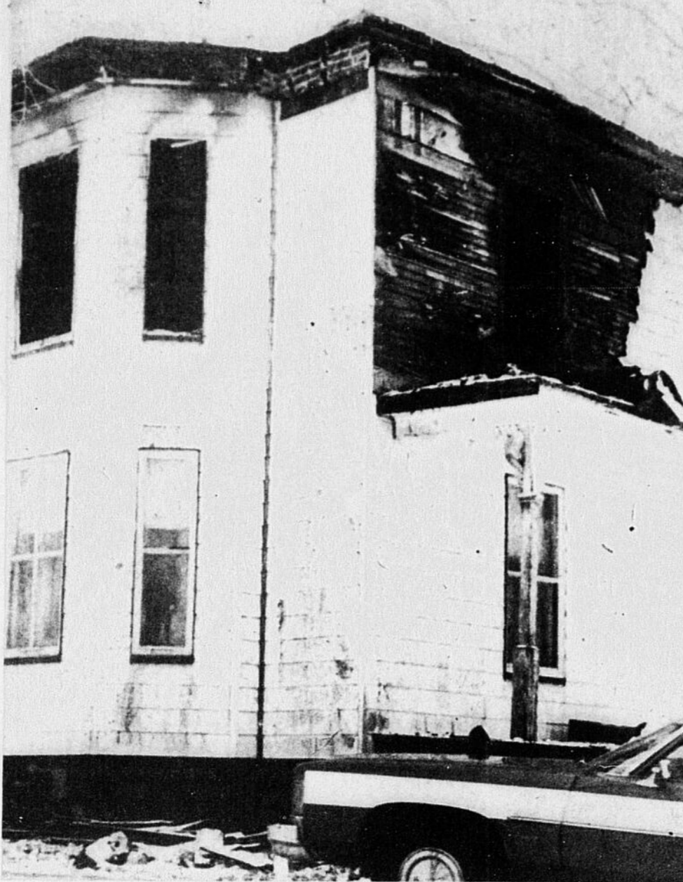
Fire damage at Arnold farm.
