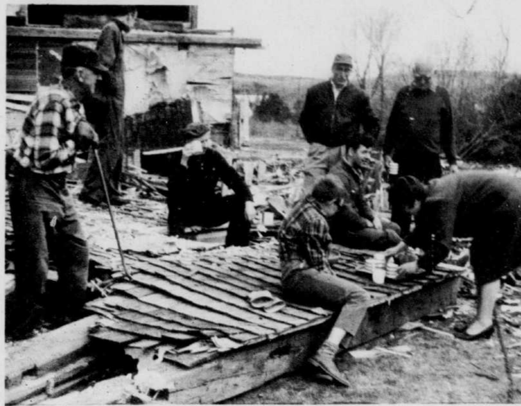
EVERYTHING STOPS FOR TEA — Mrs. R. W. Peirce, the wife of the rector of Christ Church, Stanstead, (At right) pours tea for the men of the church who stop a moment from dismantling what was the former Gibson House. The house is now owned by the church and after the removal job is complete will be levelled off for a church parking lot. In the picture, left to right are some who turned out for the tea: John Smith, Alfred Middleton, Edward Hyatt, Donald Prangle, Uisford Cargill and at the front are Michael Pierce and Edward Simpson, Jr.
