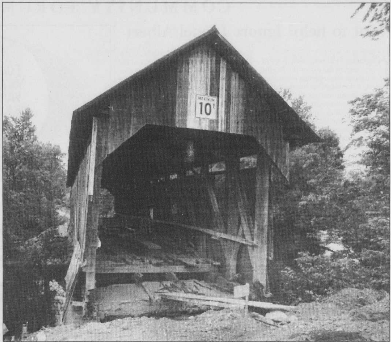
The Capelton Bridge in Hatley Township is ranked fourth out of the 91 covered bridges remaining in Quebec.
