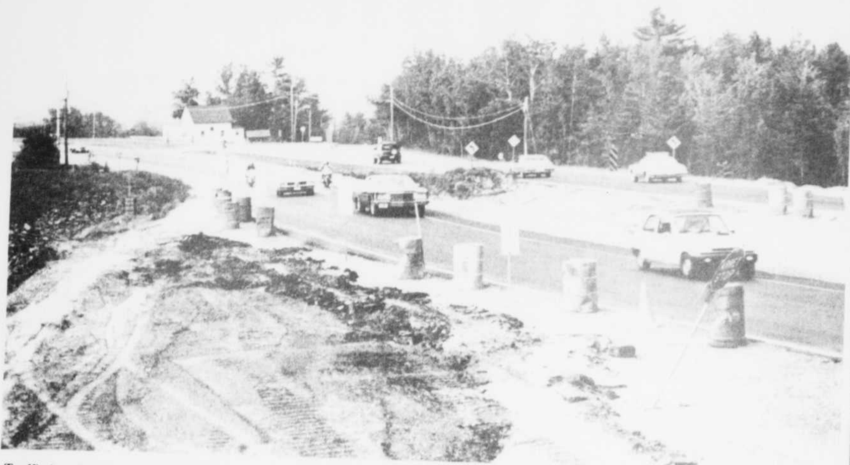
Traffic is reduced from four lanes to two west of Deauville. The detour extends as far as Omerville.
