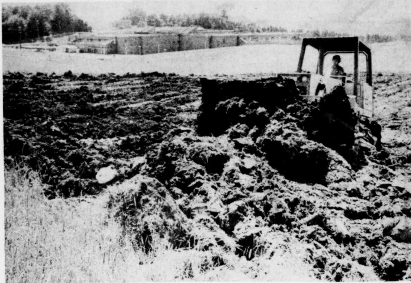
CONSTRUCTION BEGINS — View Point Development construction crews began earth-moving operations on the grounds of Alexander Galt Regional High School earlier this week. The construction work involves ditch digging to improve drainage and the expansion of the parking lots. See story pg. 3. (Record photo: James Bruce)
