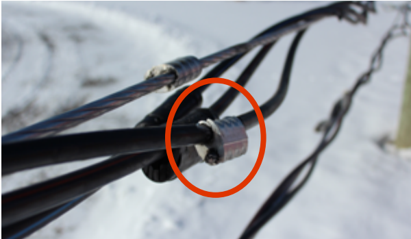
Cover missing on the connection
