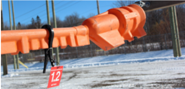
Correctly installed conductor covers
