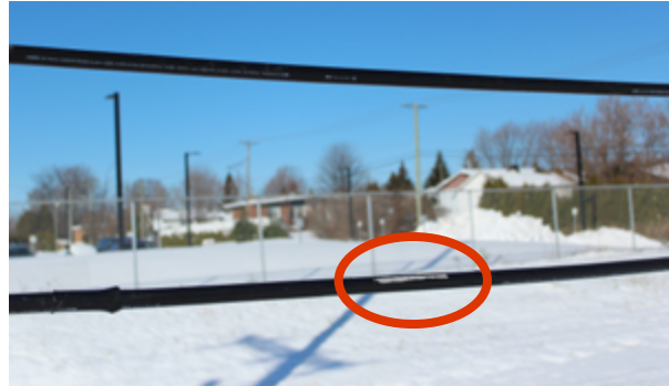
Damaged conductor sheath
