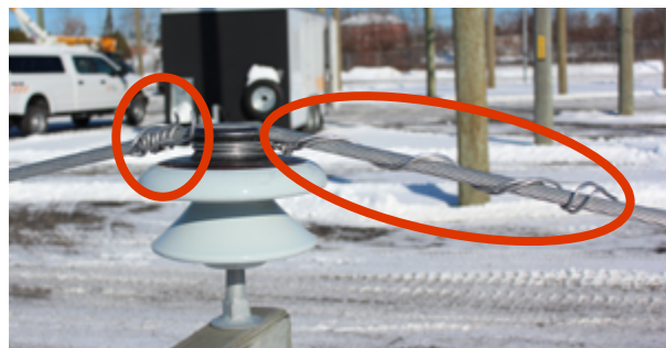
Loosened tie wires
