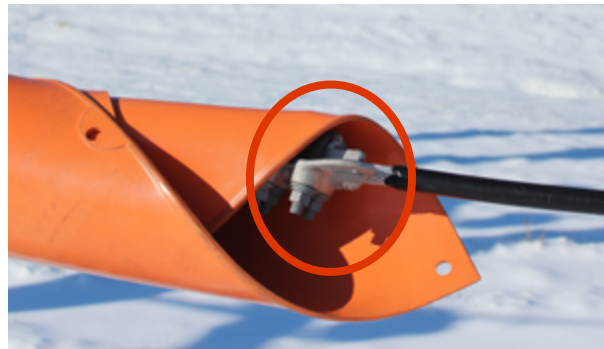
Part of the conductor is exposed
