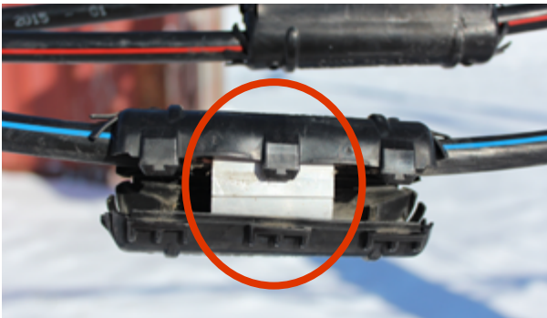
Open or damaged cover
