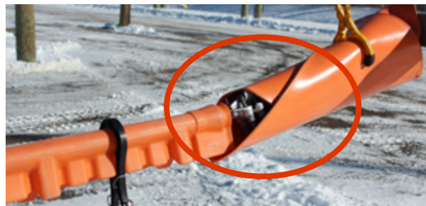
Incorrectly superposed conductor covers
