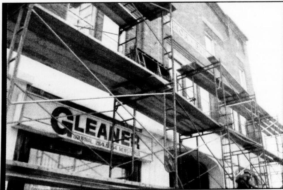
Workers have started repairs on O'Connor Building's façade. The CDC and the Town of Huntingdon recognized the urgency of the situation.
