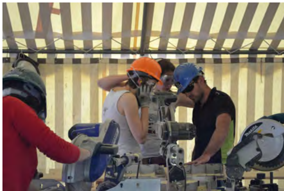
Figure 4.10 – Salle de machineries
