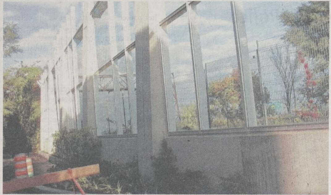
Seen here is an experimental sound barrier section at the foot of Abbott Avenue. Presently, Westmount officials are disappointed with the MTQ after several delays towards the receipt of a comprehensive sound wall feasibility study. TC Media - Examiner Photo
