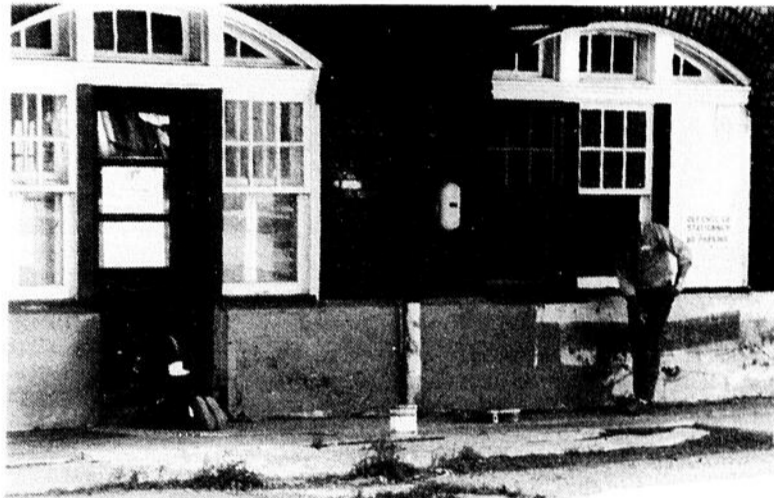
STATION SPRUCE-UP: CP Rail employees were busy Tuesday morning painting the front of Westmount station as part of a planned clean-up mentioned last week in an EXAMINER article on the deteriorating state of the station.
