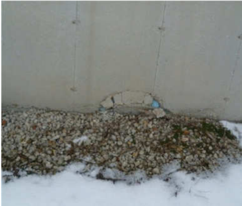
Figure 23 Broken concrete sandwich wall
