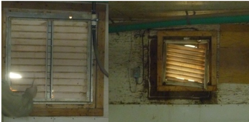
Figure 37 Damaged shutter frames that have to be replaced
