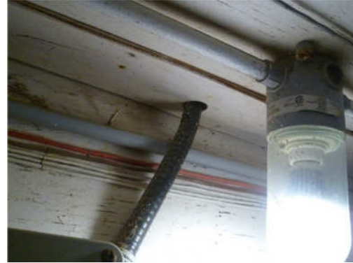
Figure 26 Perimeter of electrical wiring conduit allowing air infiltration that has to be appropriately sealed
