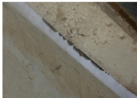
Figure 22 Caulk applied to wall-ceiling junction is coming away from the surface. It has to be removed and reapplied.
