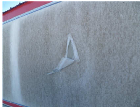
Figure 13 Damaged prefilter that has to be replaced
