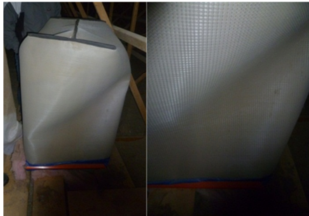
Figure 15 Dust clogged anti-microbial filters that have to be cleaned
