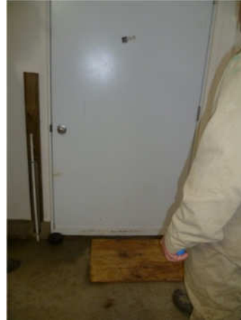
Figure 33 Threshold raised above floor and protected by a temporary wooden ramp
