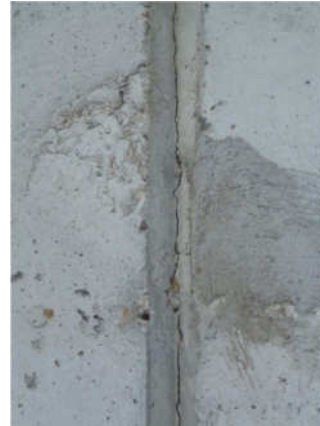
Figure 24 Sandwich wall with cracked control joint that has to be sealed with an appropriate caulk
