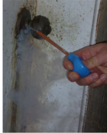
Figure 17 Smoke test showing air leakage through the screw holes of an exterior door handle
