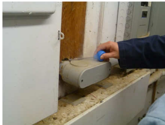
Figure 27 Infiltration of air through a hole in the wall created by a PVC conduit body. Hole has to be sealed with an appropriate caulk
