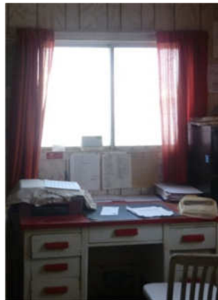
Figure 18 Office window that has to be sealed and covered with a Plexiglas panel from the inside
