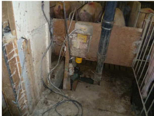
Figure 42 Reception pit submersible pump in gestation unit
