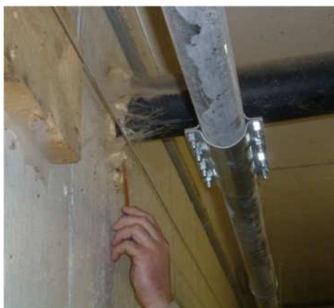
Figure 28 Smoke test done on the perimeter of a feed line sealed with foam allowing you to see that air infiltration is possible
