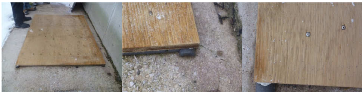
Figure 45 Airtight cover on a pump-out port
