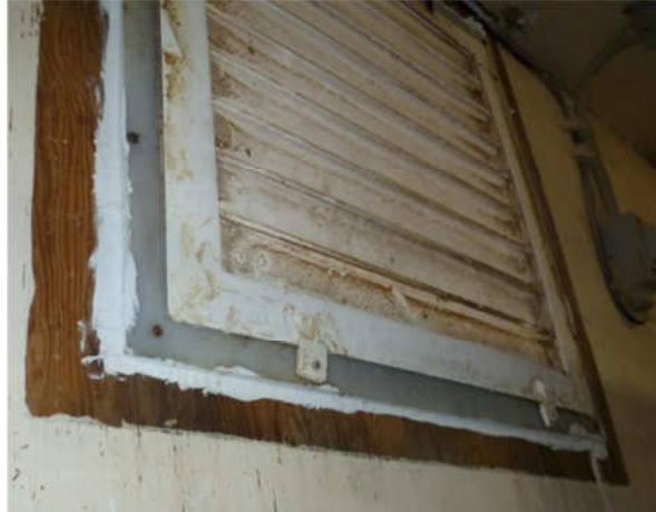
Figure 36 Perimeter of a fan housing that has to be sealed
