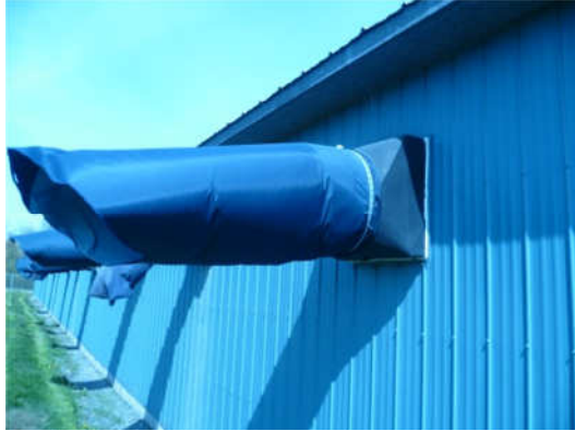
Figure 38 Air chute on vent
