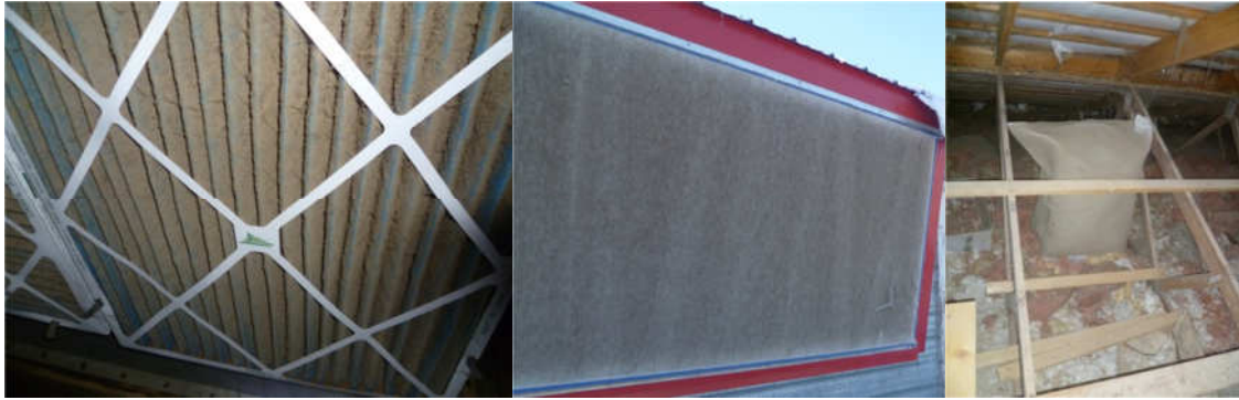
Figure 14 Dust laden prefilters that have to be replaced
