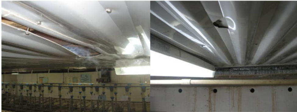
Figure 41 Breaks in corrugated plastic Manure discharge pipe Photos : Darwin Reicks
