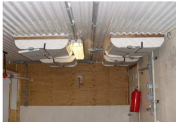
Figure 35 Conterweighted air inlets allow entry of filtered air inside a ventilated loading bay under negative pressure
