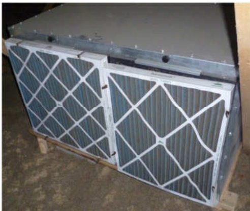
Figure 12 Prefilter not properly held in place by fasteners/clips (prefilter tends to fall when fasteners/clips are located on the sides of the prefilter)
