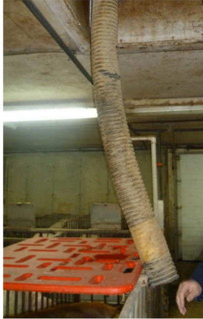
Figure 50 Possible air infiltration through the feed line from an empty feed bin
