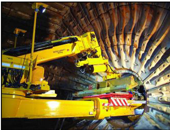
Figure 1.24: Russell technology for re-lining grinding mills.
