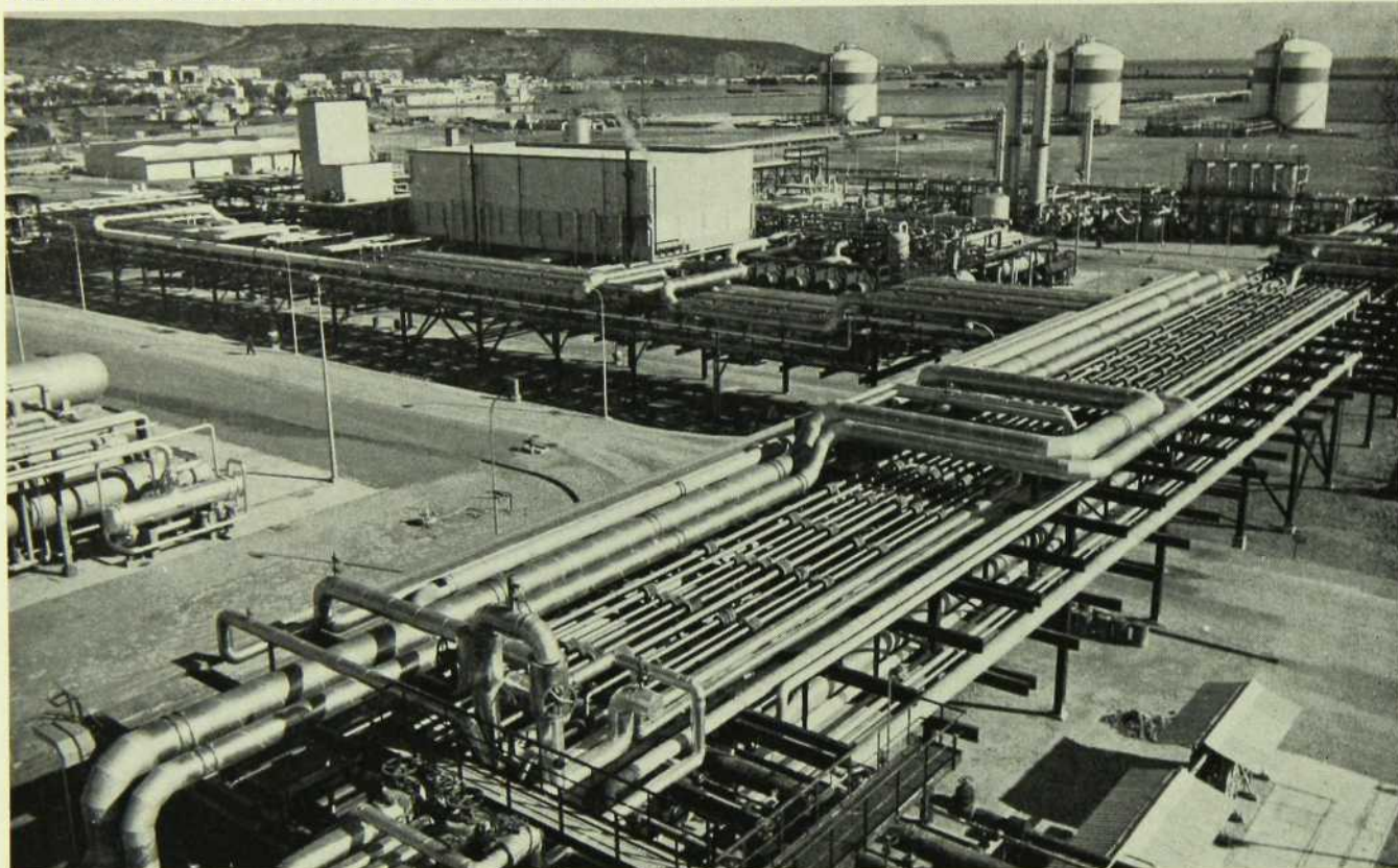
Camel's liquefaction plant in Arzew (Algeria)
