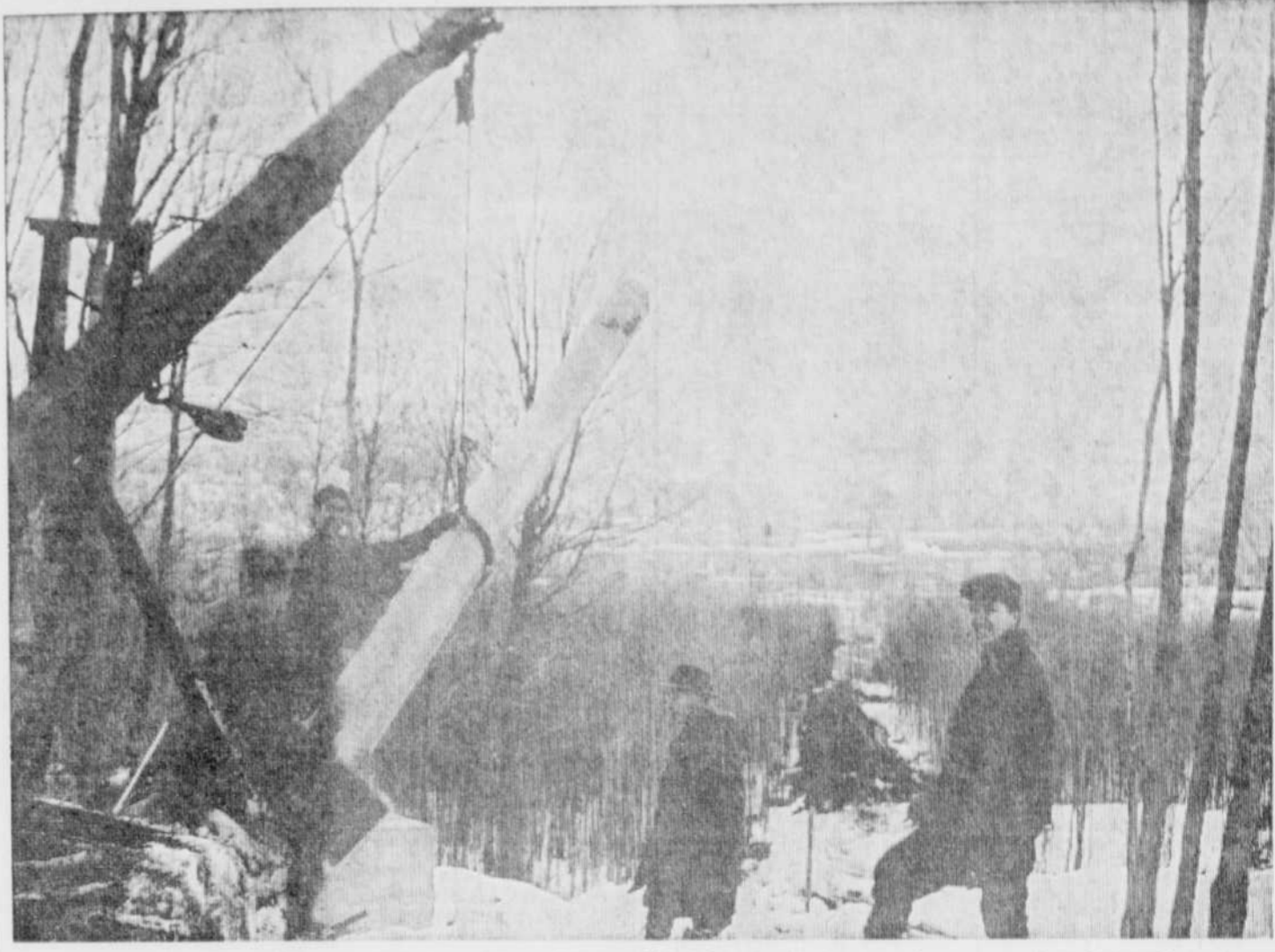
THE LAST ONE — Eric Schiller, (second from right) ski expert hired by the city to supervise construction of the ski center on the slopes of the luminous cross mountain is pictured doing just that. He is supervising the installation of the last steel pole to be installed for the installation of the $200,000 "poma lift". Installation of the lift should be completed by next week. (Record Photo by Gerry Lemay)
