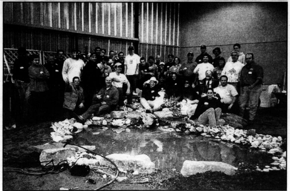
Students and instructors with the completed pond at the Career Centre. (Photo: courtesy CVCEC)
