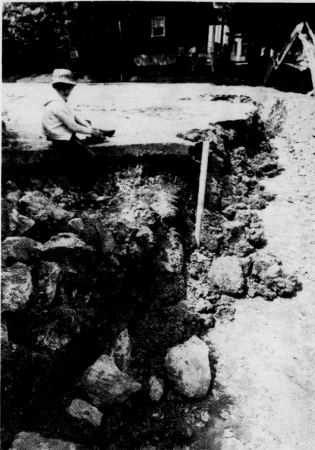
SETTING ON THE BRINK doesn't seem to bother this youngster, as he calmly sets himself down, literally on the edge of the street to empty the dirt from his shoe. The street the young fellow is sitting on runs onto 7th Avenue, which the city is presently digging up, to permit repairs to the road bed. (Record Photo by Steve Bell)
