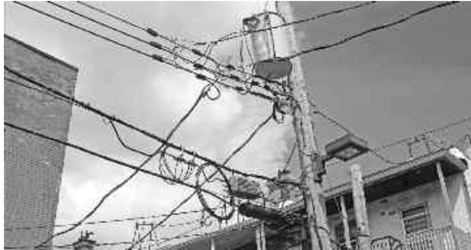
A utility pole in an alley between Prince Albert and Victoria, seen on August 19, carries cables and other electrical components from various utility companies.
