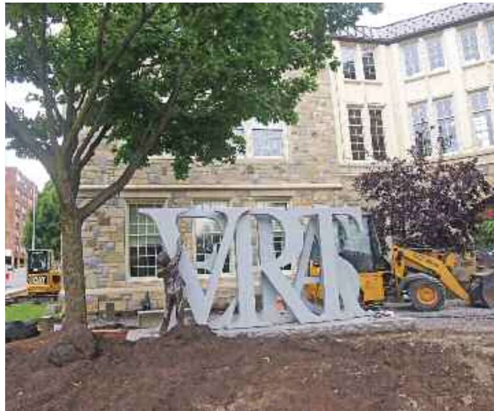
Construction for a landscaping project surrounds an preexisting art installation with the word “veritas” near the northeast corner of Côte St. Antoine Rd. and Stanton St. August 21.
