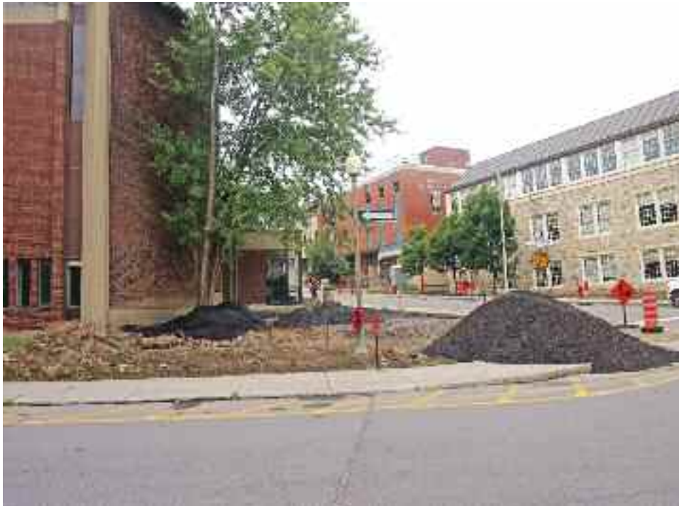
Piles of dirt lie near Selwyn House's Macaulay building at the northwest corner of Côte St. Antoine Rd. and Stanton St. August 21. Of the landscaping projects, this one "will be smaller," according to Hal Hannaford, head of school.
