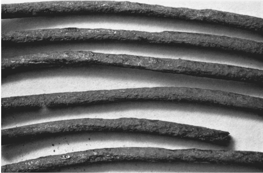
Figure A.6 — Corrosion considérable
