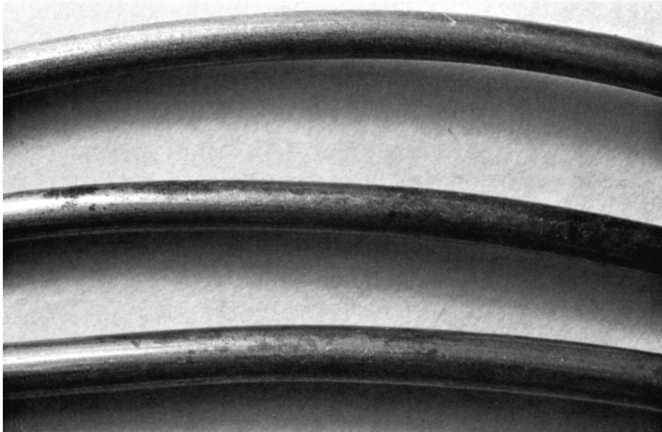
Figure A.2 — Traces de corrosion
