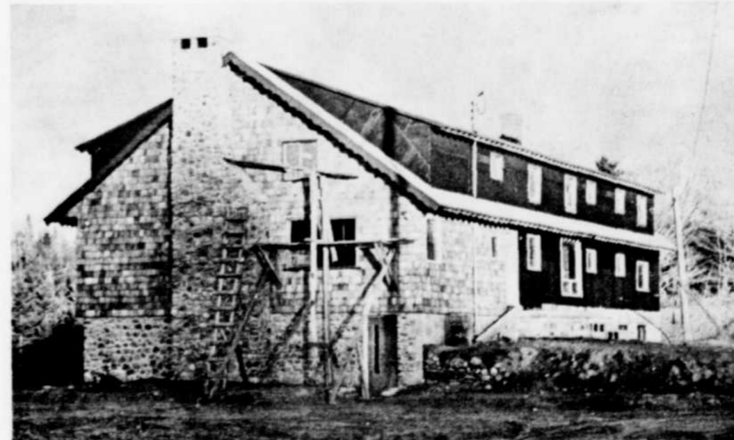
NEARING COMPLETION AT CHERRY RIVER — Parkside, a youth camp at Cherry River, run by The Christian Brethren, is close to finished. Located a mile north of the village, this hostel will be used the year round for youth groups. It's a large 2 storey structure, with the atmosphere of a country chalet, and basically intended as a religious retreat for young people. One completed, Fred Warnholtz, pastor of the Cherry River parish, and Mrs. Warnholtz will reside here as hosts. The camp is designed to accommodate some 100 to 120 young people at a time. (Photo: Charles Catchpaugh)
