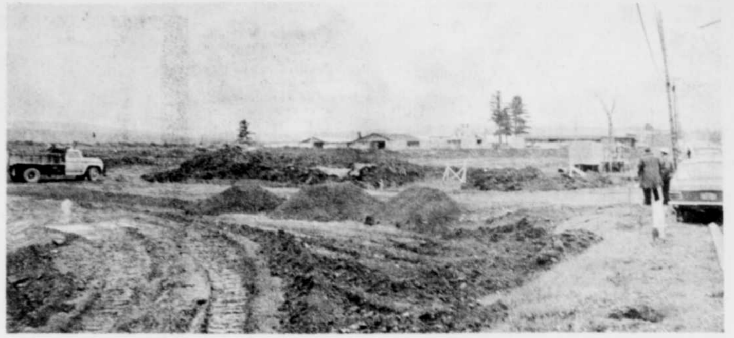
WORK BEGINS FOR NEW MAGOG PLANT — There is plenty of activity in Magog's industrial park, where Montreal Offset Ltd. has begun. Site of the operation, pictured above, is on Sherbrooke St. (Photo: Charles Catchpaugh)
