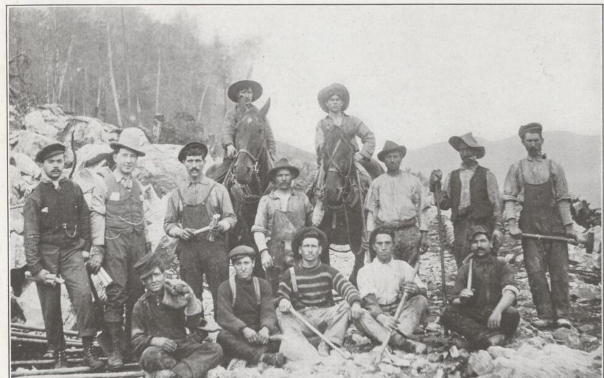
MONTREAL REACHES OUT INTO NORTHERN QUEBEC—A construction gang on the Nominig-Rapide de L'Original branch of the C.P.R. (Photo by H. Richards.)
