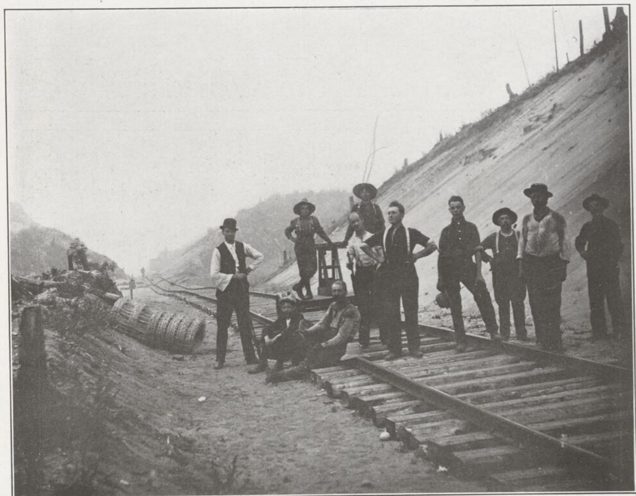
MONTREAL REACHES OUT INTO NORTHERN QUEBEC—A section gang straightening and levelling the newly-laid track on the Nominig-Rapide de L'Original branch of the C.P.R. (Photo by H. Richards.)
