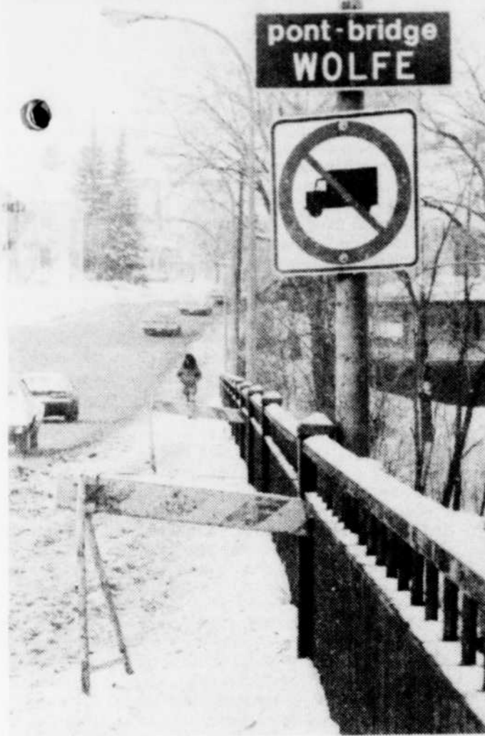
NO HEAVY TRAFFIC — That includes pedestrian traffic too! This section of the sidewalk on the Wolfe Bridge has been cordoned off because parts of the concrete have fallen away.
