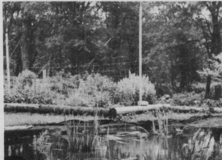
Large stones and edging plants cover the thick felt and PVC liner of this new garden pool. The excess material will be cut away.
