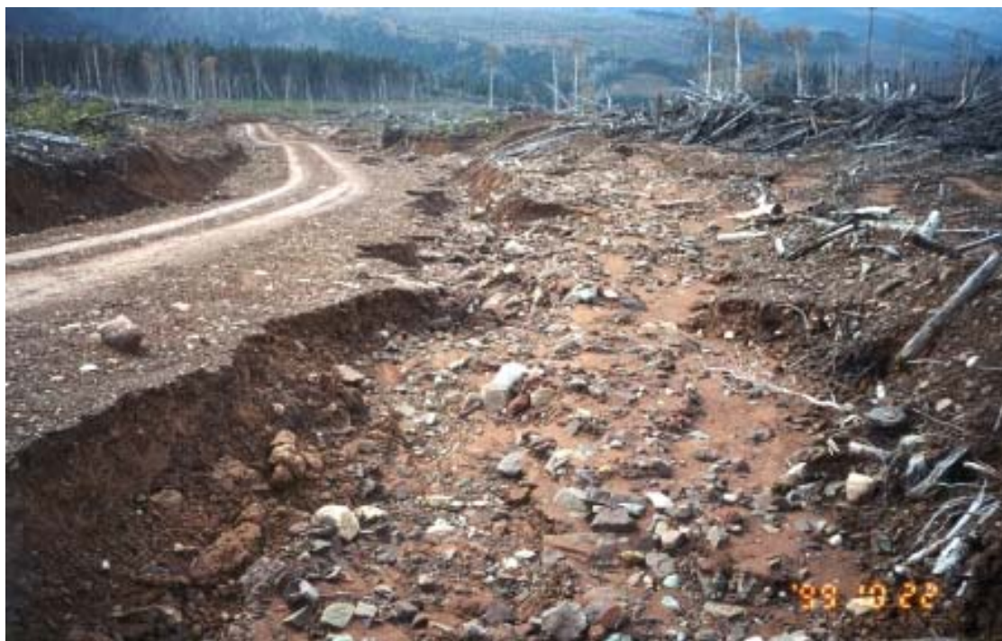
Erosion of ditches along a forest road
