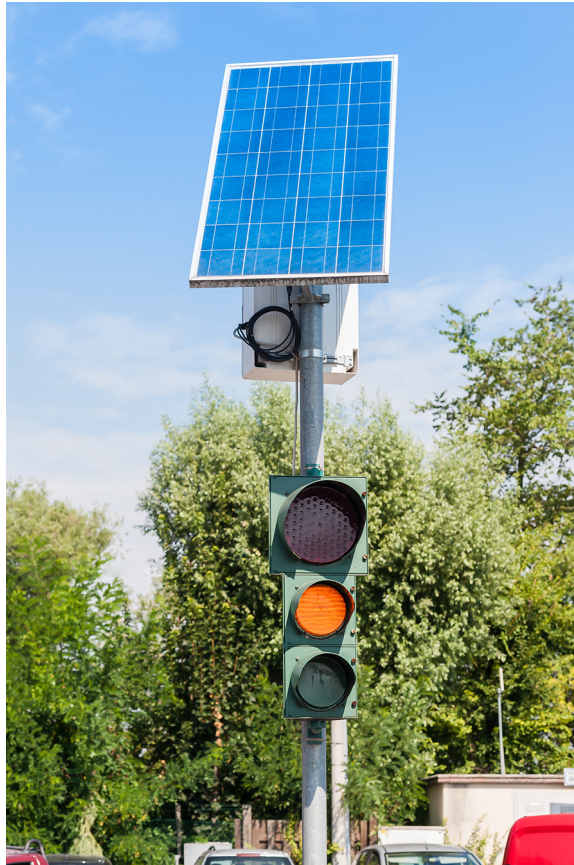
Figure 21. Solar-power traffic lights.
