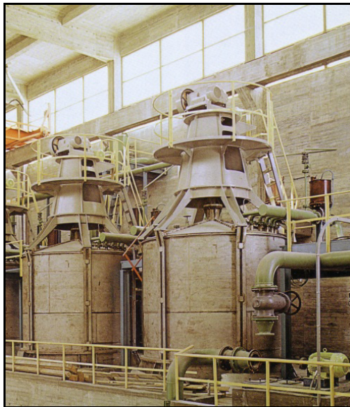
Figure 3.33: Cooling vessels to crystallize calcium nitrate tetrahydrate.
