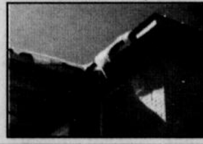
It's very important to inspect the outside of your home before the winter arrives.
