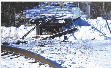
There is a history of ice dams washing away bridges in the Saint Francis Valley, but it is quite a different thing to see the remnants outside the pages of a textbook, as happened last January in Bromptonville.
