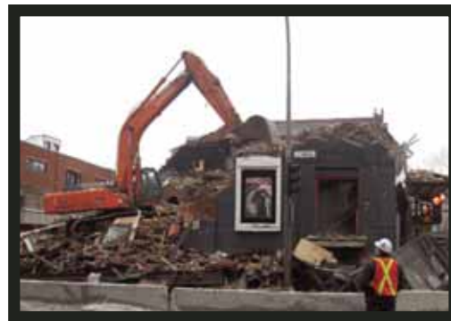
Demolition of the old Théâtre de Quat'Sous before its reconstruction, February 2008 © Eric Jean
