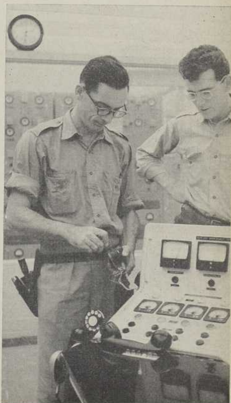
BELL MEN INSTALL ONE OF THE NEW EMERGENCY INTERCOM PHONES IN THE NRX CONTROL ROOM.
