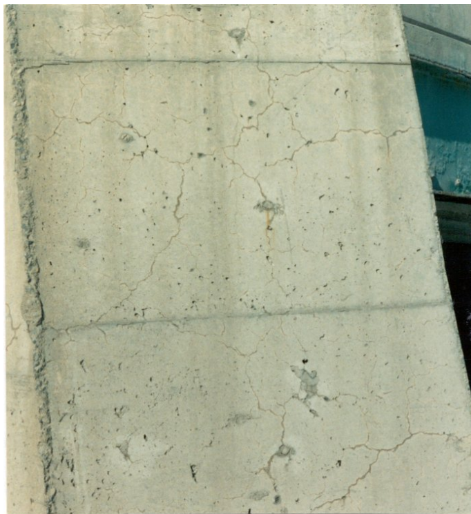
Photo 4.2-5 d) Fissures polygonales
