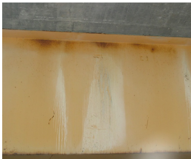
Photo 10.3-2 Points de corrosion
