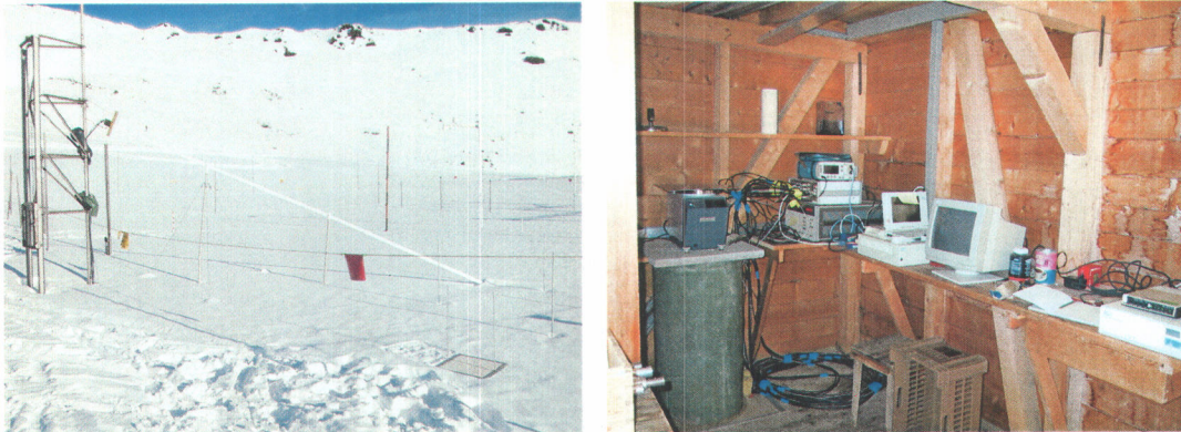
Figure 3 - The cable sensor system at Weissfluhjoch Davos (2550 m): the sloping flat-band cable (left), and the electronic devices in the shelter (right).
