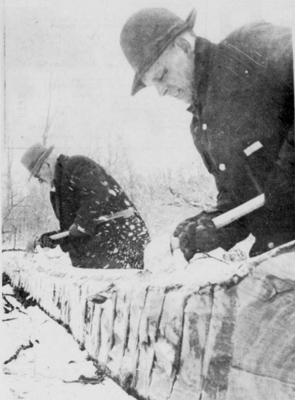
HOME STEAD RESTORATION—Simeon Martin (left) uses the adze and the broadaxe to square up timbers for the authentic restoration of an
