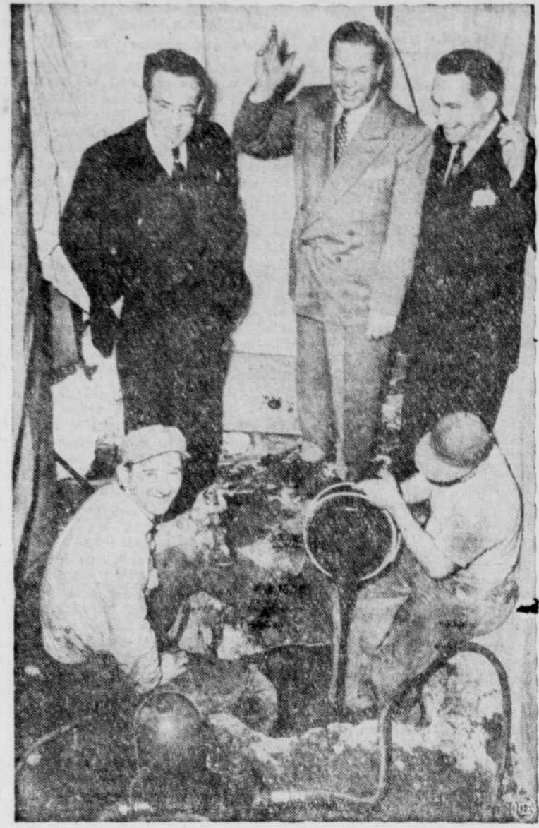
To water-short New Yorkers the finding of a new water supply is cause for rejoicing. Here, officials of the Ambassador Hotel are all smiles as they watch workers tap an old, unused well in the hotel's basement. The spring was used by a brewery once located on the site.
