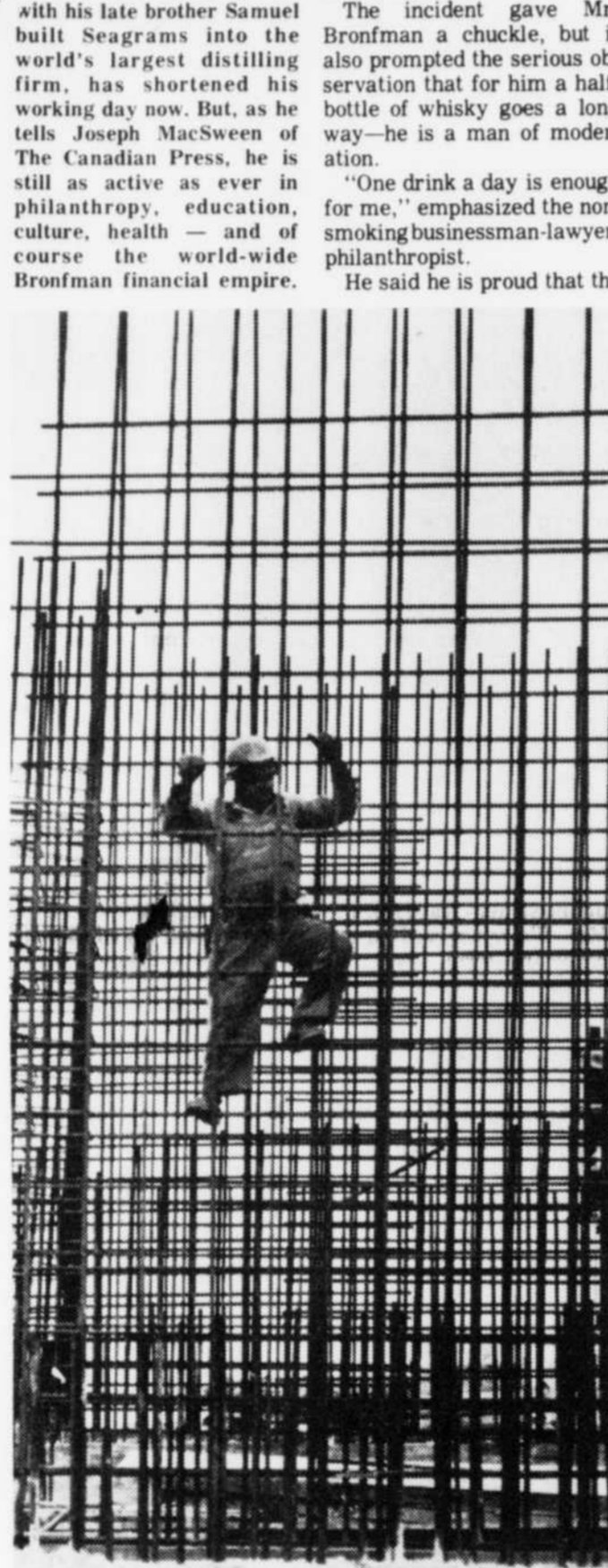
WEB OF STEEL surrounds a construction worker at Hibbing Taconite Co.'s iron ore plant near Hibbing, Minn., as he inspects foundation reinforcements at the site. When completed, the plant will produce 5.4 million tons of high-grade iron ore pellets a year.
