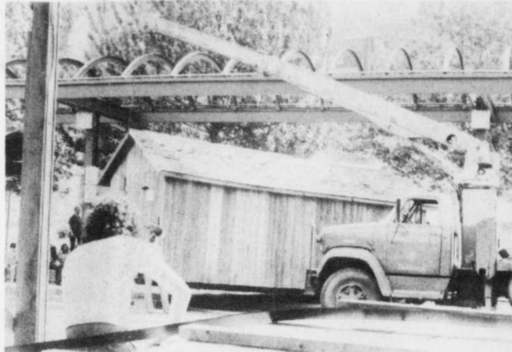
GETTING READY — Work crews moved in the maple sugar cabin, yesterday afternoon on Wellington Street. The building is just one of many on downtown
