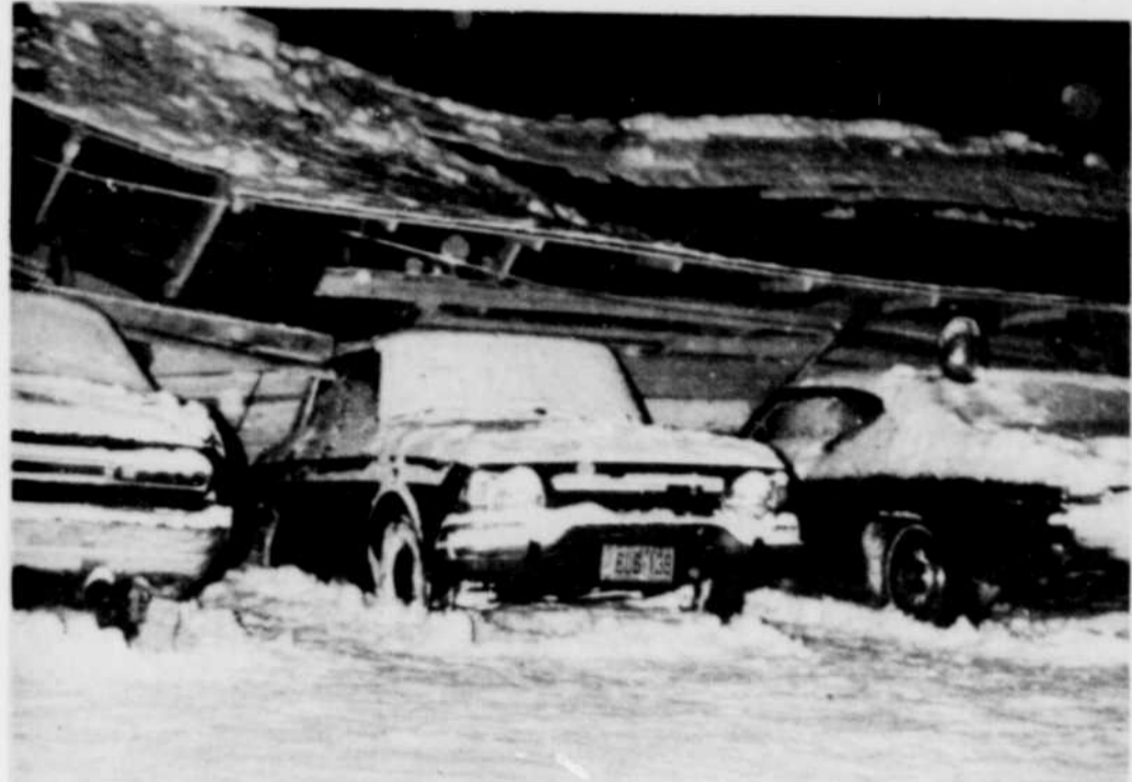
AND THEN THE ROOF FELL IN — The roof of the Torrington Company store on Reid St. in Bedford collapsed under the weight of heavy snow. Cars parked nearby were severely damaged. (Photo: Charles Nashville)
